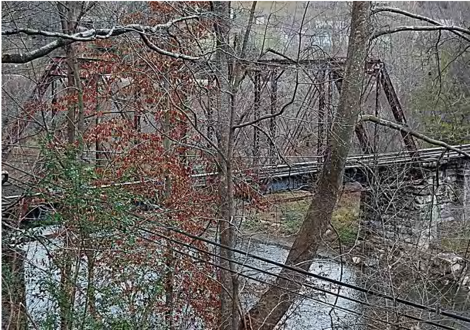
Plate 23. Murphy Branch, Pratt Truss Bridge over Valley River (Plate 22), Looking Northeast from Tennessee Street (Joe Brown Highway), Murphy.
