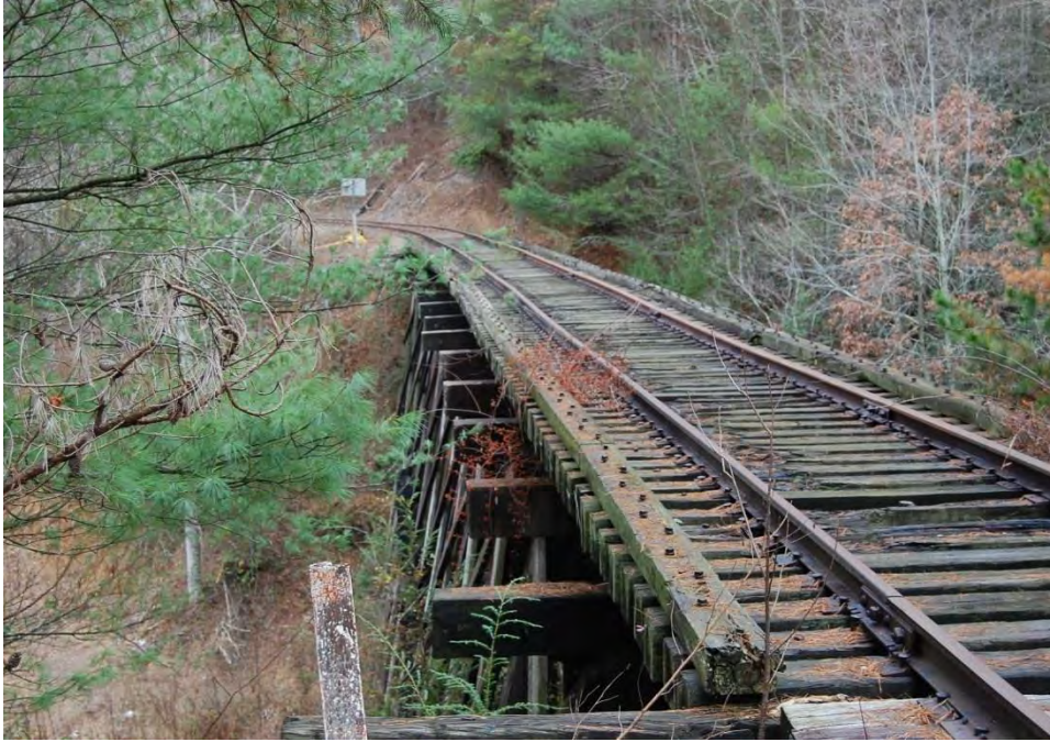
Plate 18. Murphy Branch, Railroad Bridge over Valley River, East of Ramsey Street, Looking West, Murphy Vicinity.
