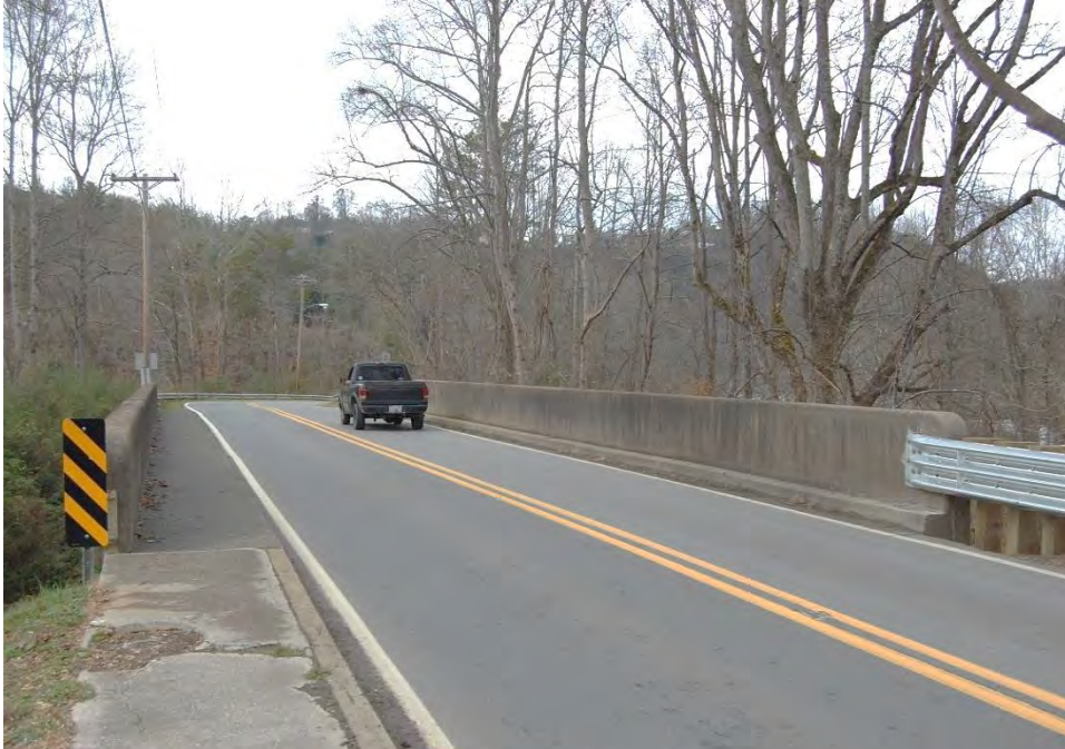
Plate 24. 1940 Reinforced Concrete, Tee Beam Highway Bridge carries Tennessee Street (Joe Brown Highway) over Murphy Branch, Murphy, Looking North.
